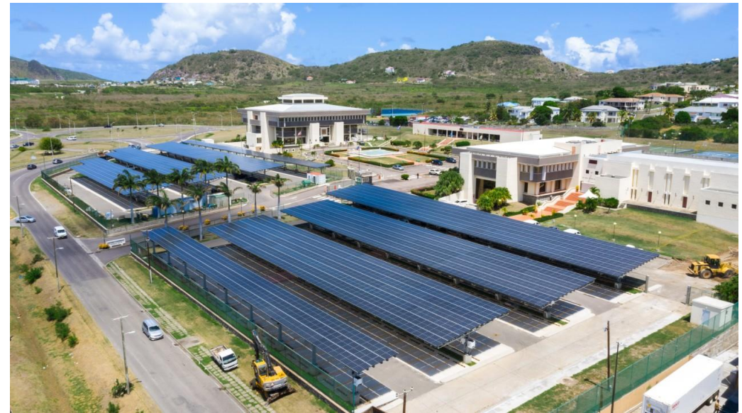
A 1.2MW solar carport located in St. Kitts at the Eastern Caribbean Central Bank, engineered to withstand a Category 5 hurricane. There could be good potential for similar structures around Bermuda. © Azimuth Energy
